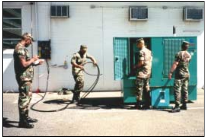
Soldiers from 249th Engineer Battalion hook up a 35 kilowatt generator outside of the Corps' Emergency Operations Center in building 230 during the statewide Makani Pahili hurricane preparedness exercise May 8-12. Photo by Alexander Kufel
