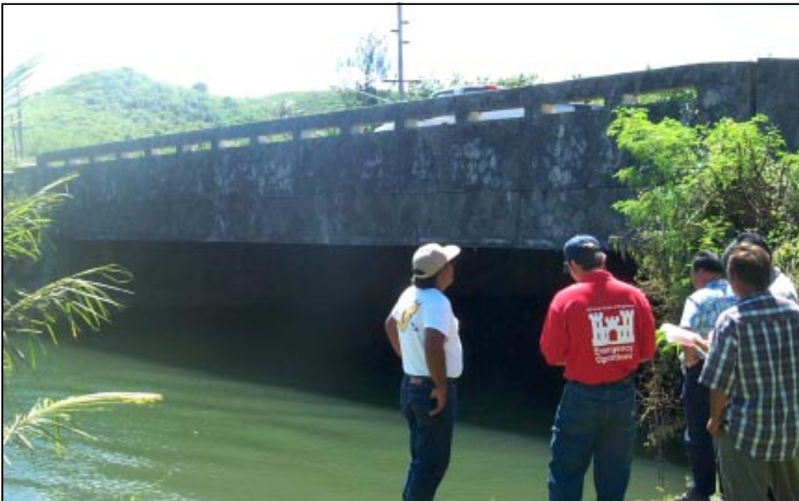
David Okada, HED Design Branch civil engineer, does a preliminary damage assessment of the Pago Bay Bridge with representatives of the Guam Waterworks Agency. The bridge sustained damage to a water main during an earthquake that struck the island on October 13. —Photo by Don Yorimoto.
