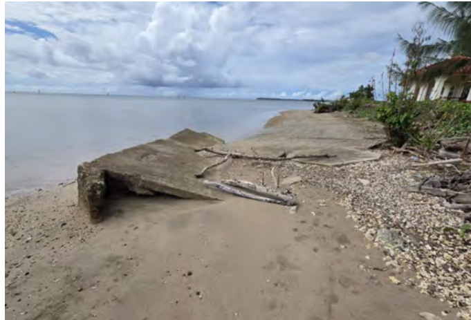
Figure 4 Erosion at north end of Nimitz Beach as of Sep 2025. Sidewalk has eroded into the shoreline. (USACE 2025)
