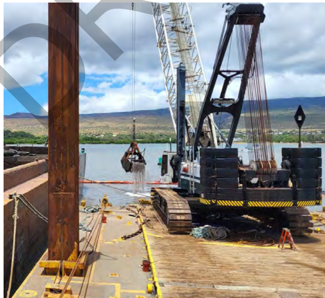
Figure 15 Example Mechanical Maintenance Dredging, Kaunakakai, Molokai, Hawaii by USACE. Mechanical dredge staged atop dredge barge in foreground, active dredging in corral, dredged material scow abutting barge to left.
